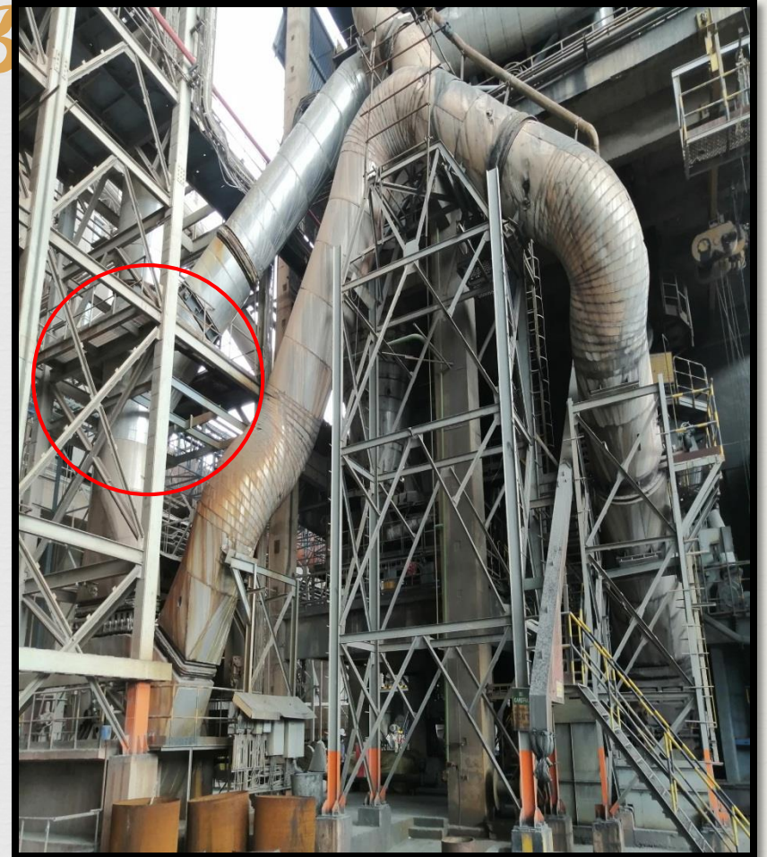
Hot gas duct joining coal mill-2 inlet duct
