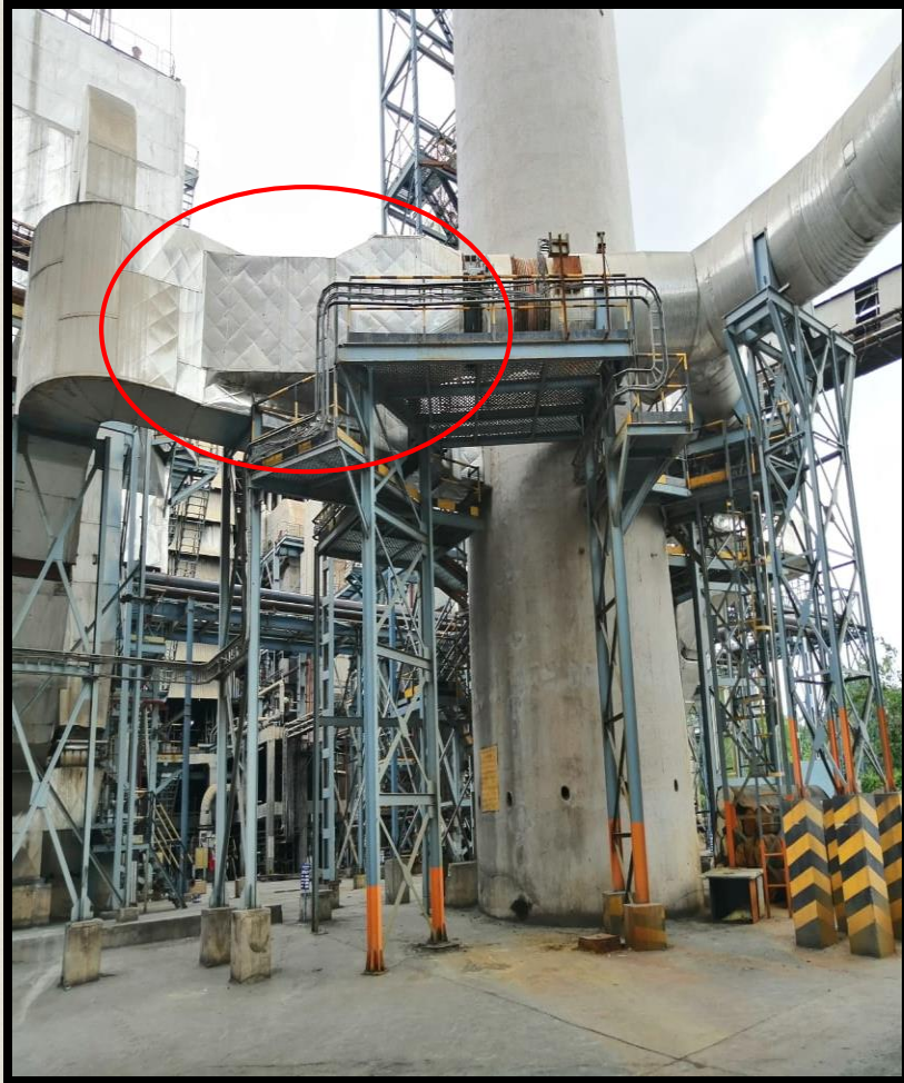
Hot gas duct from TPP
